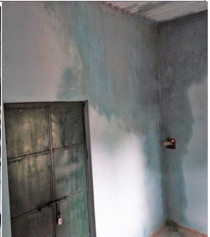
Seepage in the newly constructed PMAY-G house, Odisha
