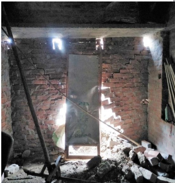
The wall of the PMAY-G house fell down in heavy rain due to non-plastering, Uttar Pradesh.
