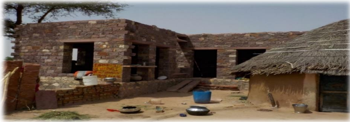
Photo 4.2: An incomplete PMAY-G House shown as Complete in AwaasSoft
